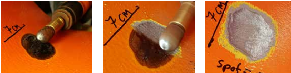
Corroded surface before and after treatment
