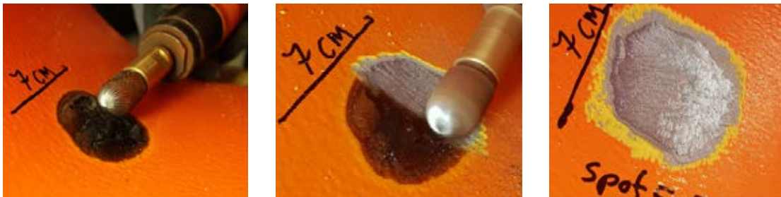
Corroded surface before and after treatment
